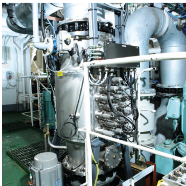
PureBallast 3.1 reactor integrated into pipework after installation
